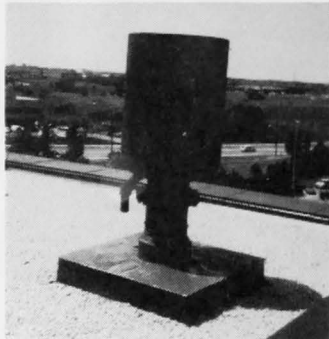
The radome base contains one of the roof's strangest objects — an ugly brown container resembling a dinosaur's drinking cup. It's used as a spare exhaust for the boiler room.
