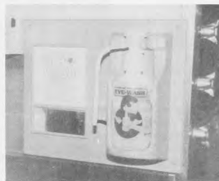
A further safety measure is the provision of eye wash fluid in a specially marked container just in case some corrosive chemicals are accidentally splashed.
